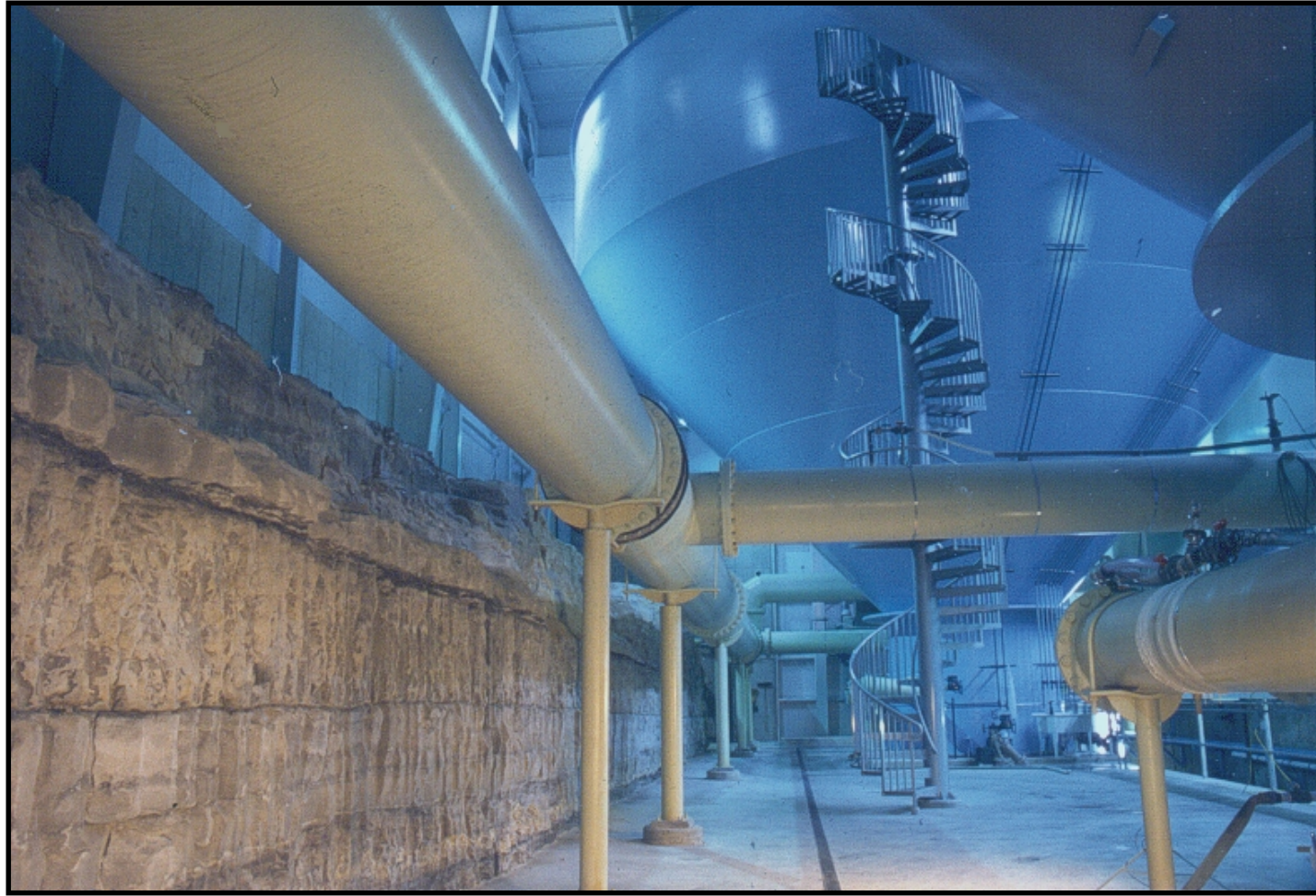
Mississippi River water is pumped through a network of pipes into massive cone-shaped clarifiers where sediment and dissolved minerals are removed from the swirling water. Keokuk's expanded, state-of-the-art water plant includes a 12-ft-high portion of the 345-million-year-old Mississippian limestone bluff along one entire interior wall of the 300-ft-long building.
