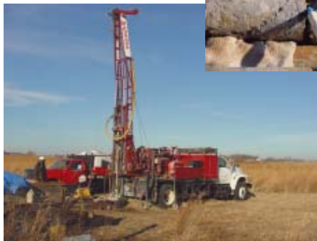
Drilling the Rutland Marsh monitoring well in Humboldt County. Close-up shows fractures and pores within the rock.
